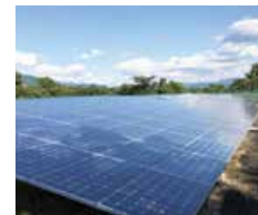
S-08 Shinshiro Solar Power Plant
